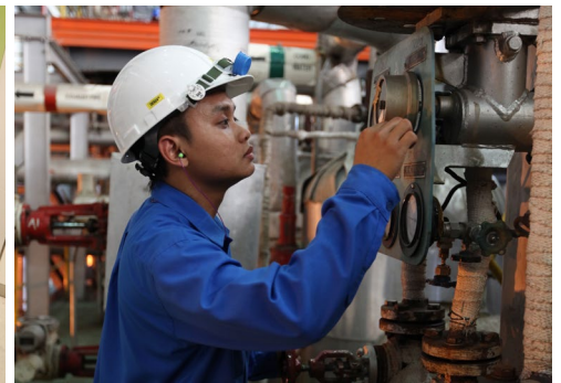
Maintenance technician inspecting power plant equipment at Sejingkat Power Corporation
