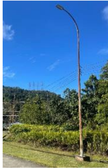
Photo 68: Corrosion on the streetlamp pole due to H 2 S
