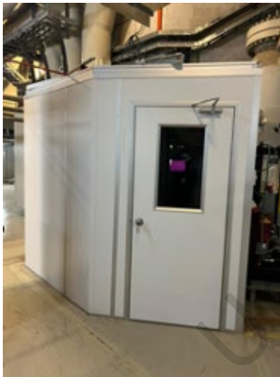
Photo 70: Seclusion of important equipment at Bakun powerhouse
