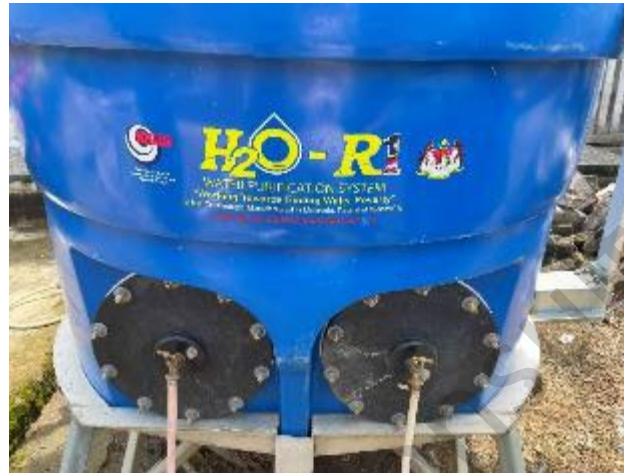
Photo 62: Water filtration system at Punan Bah
